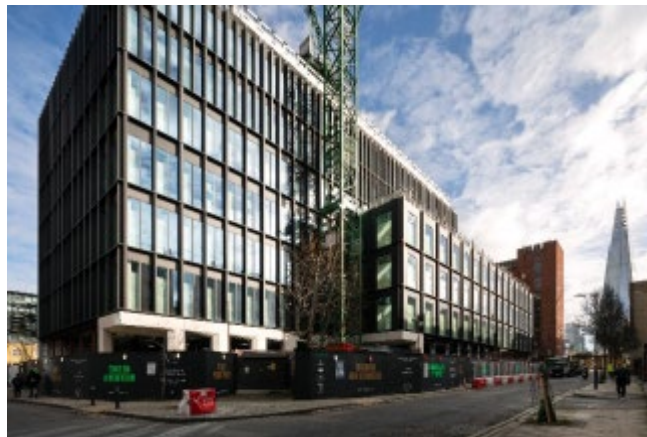
7 South and West façade elevation nearing completion (Bronze building). ©Bryden Wood. Photography by Jocelyn Low.
