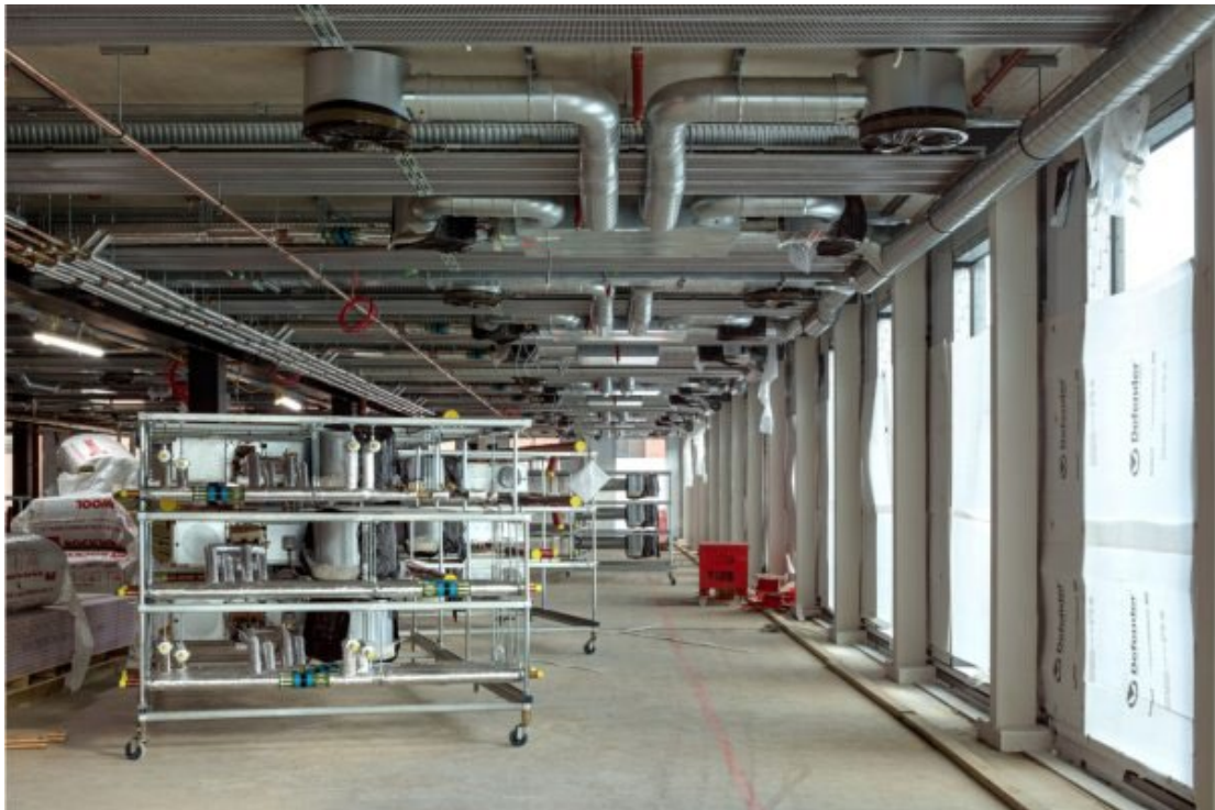
6 Floorplate with M&E cassettes fitted in position (note fan coil unit rack on its wheeled base in the foreground). ©Bryden Wood. Photography by Jocelyn Low.
